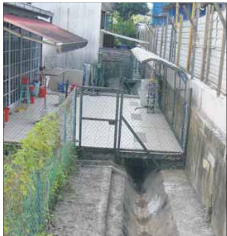
NO MOSQUITOES FOUND HERE: The gratings on the extended area can be opened to inspect and clean the drain.
